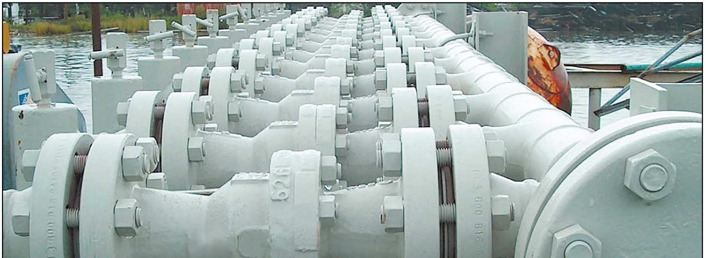
PBV® Flanged Floating Ball Valves installed in a typical manifold application.
